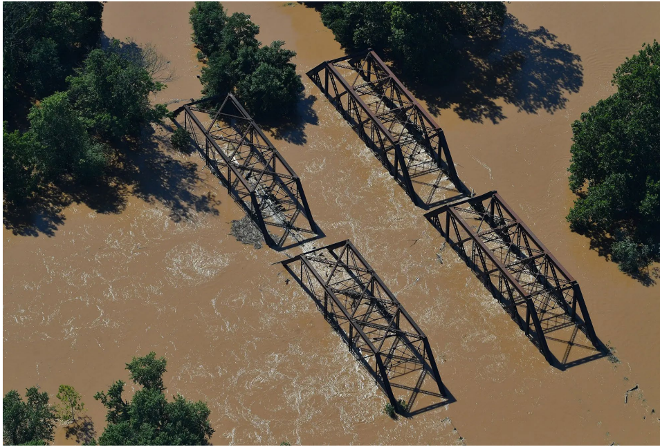
Figure 15 : Bridge in Somerset County Inundated by Floodwaters
